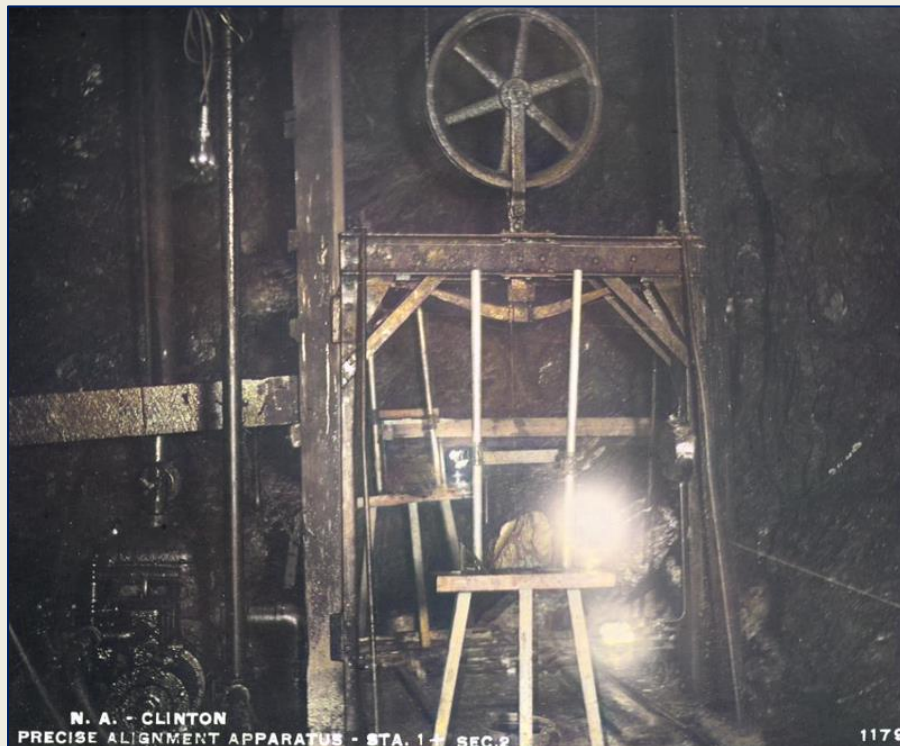
Precise alignment apparatus below Shaft No. 1.
