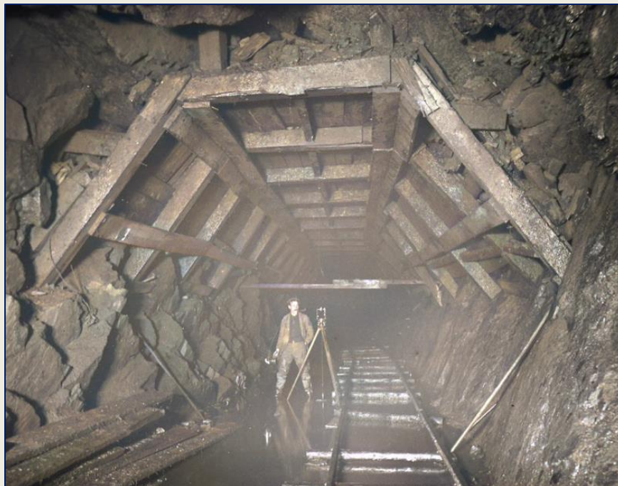
Loose blasted rock at tunnel heading.
