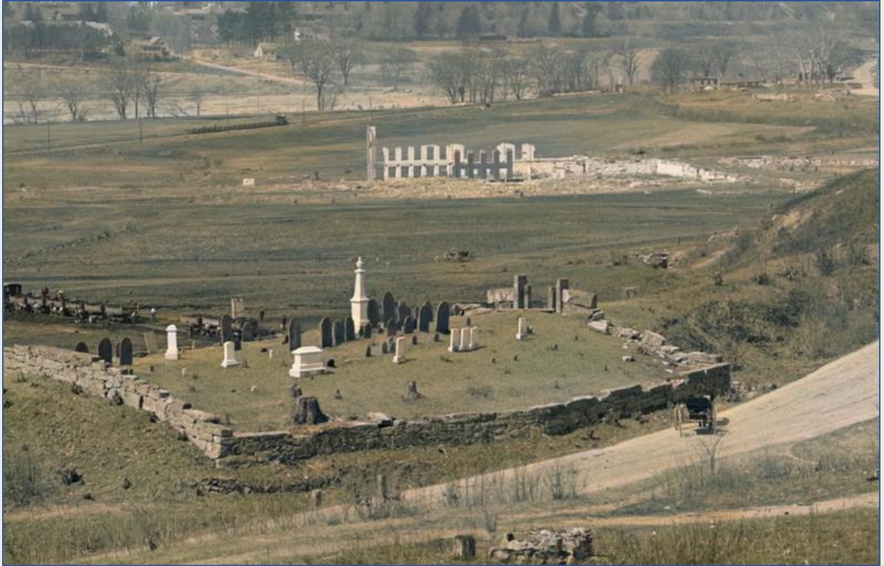
The race is on to complete the demolition and remove the debris. April 22, 1904
